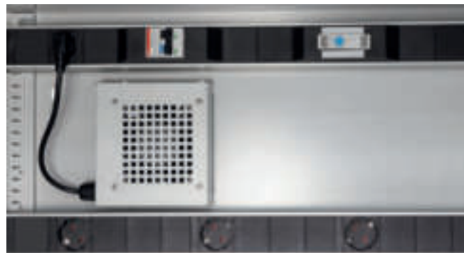
Temperature-controlled fan and central master bar in the comfort cabinet
